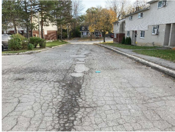
Figure 4 - Previous roadway condition at Limberlost
